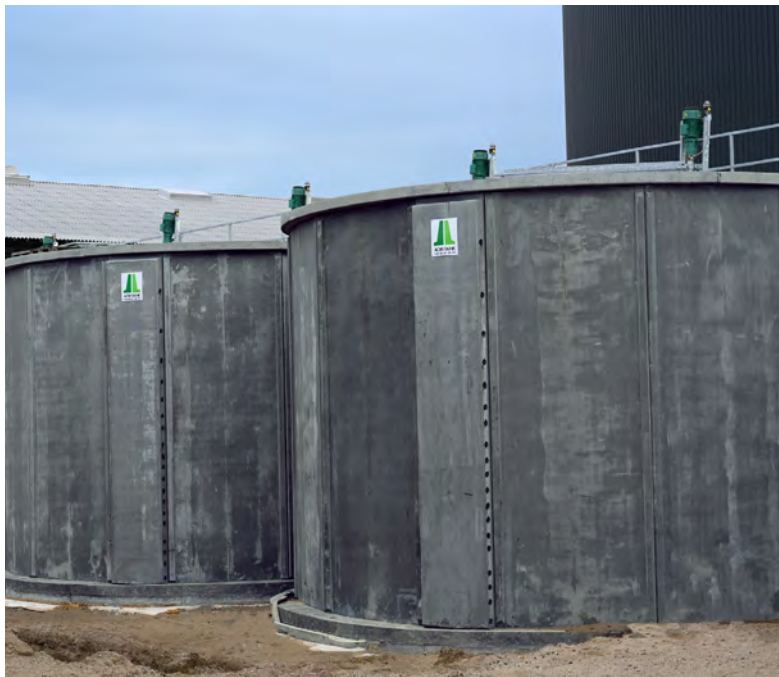
BG2 top mount - Concrete tank
