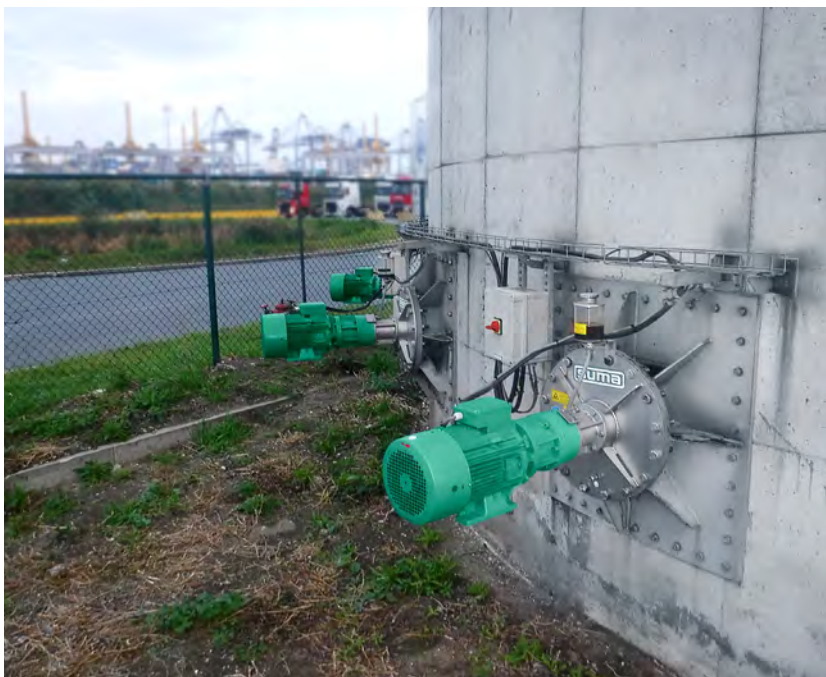
FR light - Concrete tank
